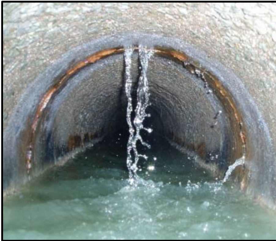
Infiltration (Groundwater via physical defects)
